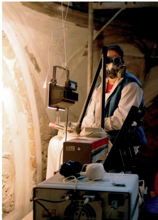
Fig.3.9.5. a) – Removal of encrustations in an enclosed room inaccessible to the public, Dubrovnik, House of Rectors. The operator is wearing goggles and a dust mask. Photo by A. Koss. b) - As in fig. 3.9.5a), operator is wearing glasses and a dust mask, Sigismund's Chapel, Wawel. The place to be cleaned is well-illuminated. Photo by J. Marczak.
